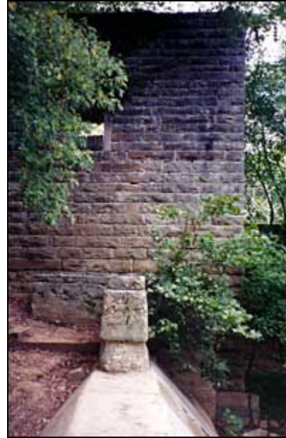
Old Mill, sans roof (tornado damage)
