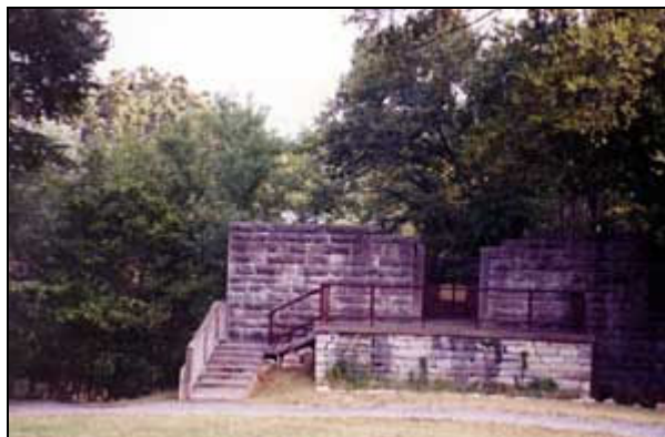
Old mill, showing tornado damage
