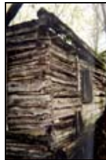
Side of small cabin; the roof is almost gone.
